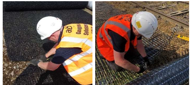
Fig. 9: Cut vegetation liner and geogrid from roll to design length using safety knife / wire cutters
