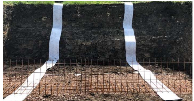
Fig. 8: Where specified, fix Fildrain to the top and down the back of the excavated slope
