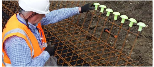
Fig. 7: Use rebar safety caps on exposed ends. A half round section of PVC pipe could also be used
