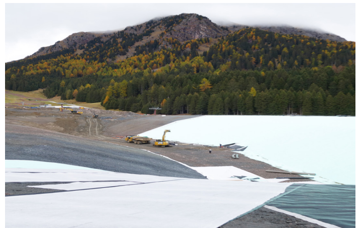
The completed accumulation basin at the foot of the Ces Valcigolera ski run, San Martino di Castrozza
