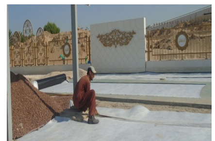
Installing the Salt Break ensuring the overlaps of filter geotextile prevent cover soil entering the capillary break void and causing tracking
