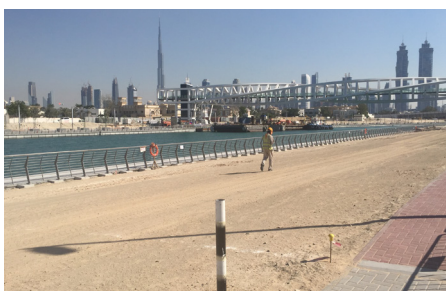
ABG Salt Barrier installed underneath landscaping running along the side of the canal
