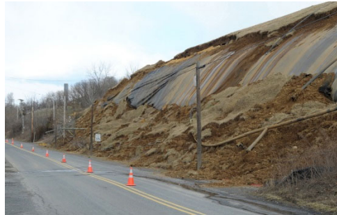
Figure 4: Translational Failure at a landfill site
