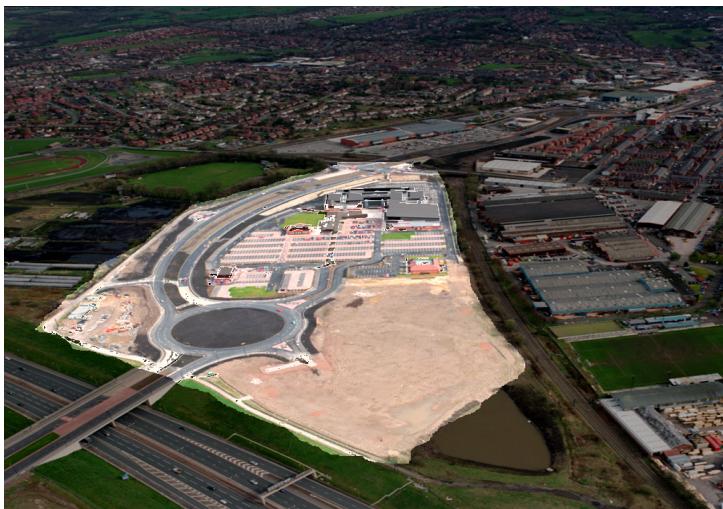
Saturated arisings from M60 cutting stockpiled and used in highlighted area with Fildrain reducing consolidation time by 80%
