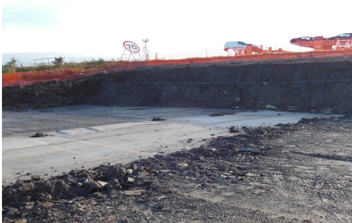
Adjacent traffic on A8 whilst locally won fill is rolled directly onto the Fildrain starter layer
