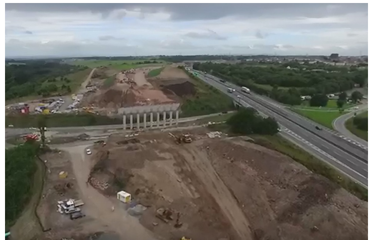
Embankments are raised along the A8 ready for upgrading to Motorway status
