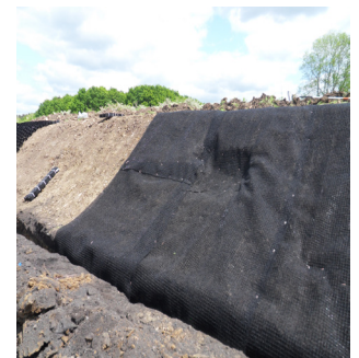
Fig. 5: Ensure Erosamat is in close contact with the ground IN ALL PLACES
