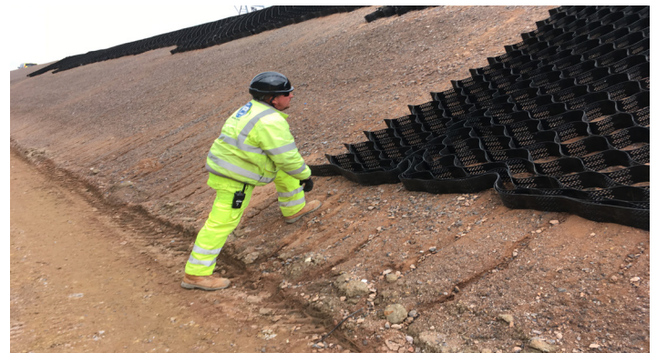
4m x 6m Erosaweb panels being expanded into position down the slope
