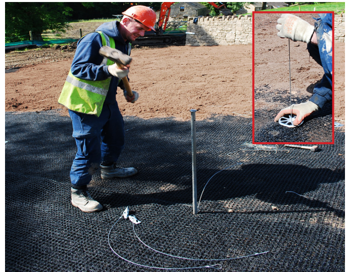
Ground anchors driven through soil. Washer placed over cable and tensioned against the geogrid.
