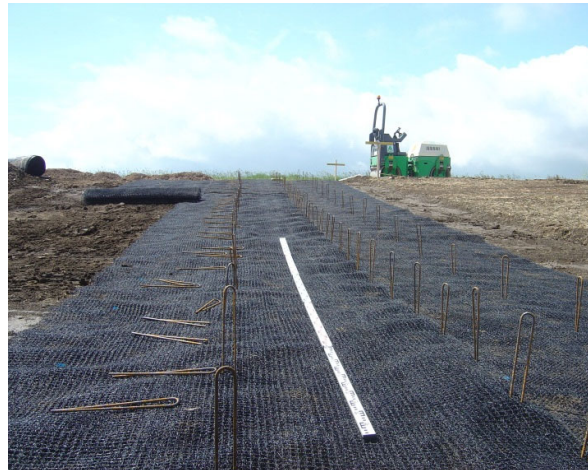
Correct surface preparation and pinning are essential to maintain good surface contact with the underlying soil followed by careful seeding and filling.
