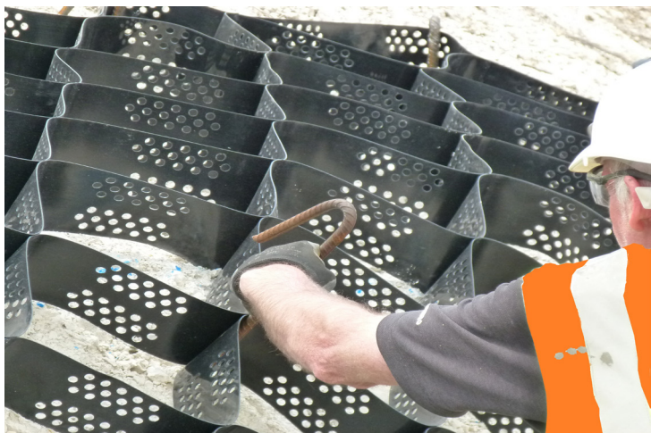
Steep, dry, barren chalk face covered with Erosaweb held with "J" pins ready to receive 150mm topsoil
