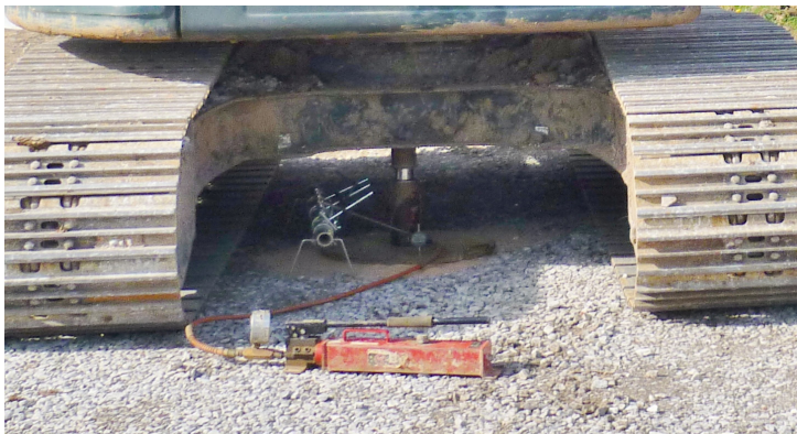
Testing after installation verified the required CBRs were achieved with the reduced material use
