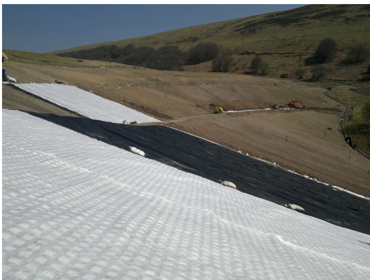
Pozidrain G with drainage in all directions placed on top of 1mm LLDPE textured liner
