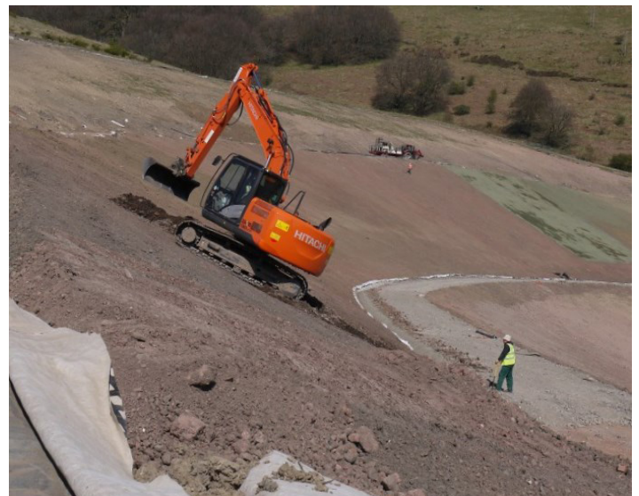
Proving high friction as construction traffic spreads cover soil, whilst protecting the geomembrane
