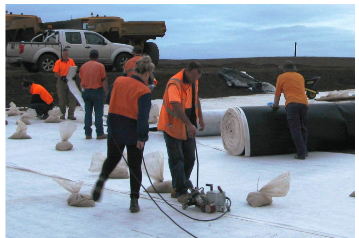
Tack welding of the geotextile overlap with a Leister gun to ensure that the rolls remained in place whilst backfilling
