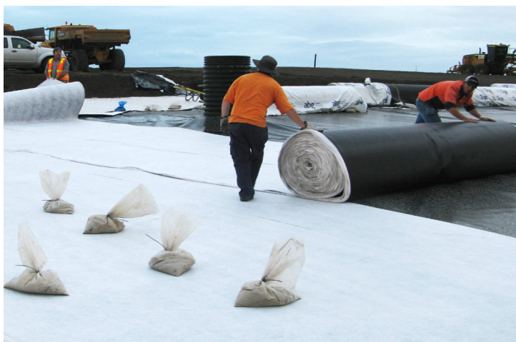
Large rolls butted together on top of the geomembrane with a geotextile overlap at the edge ready for tack welding
