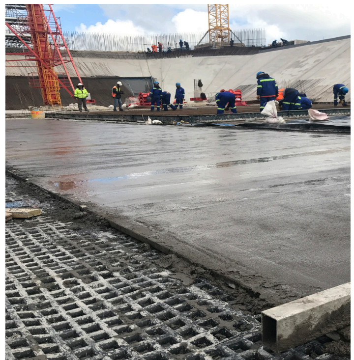
Screed cast into the Leakdrain cusps beneath HDPE slip and water stop channel layers.
