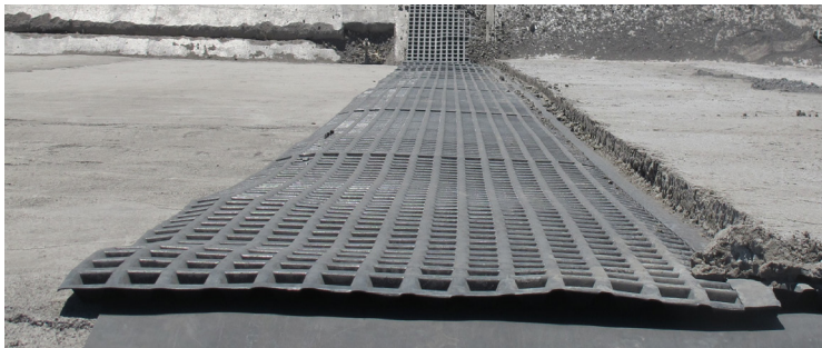
Leakdrain providing the void space and additional protection barrier above the secondary HDPE liner.
