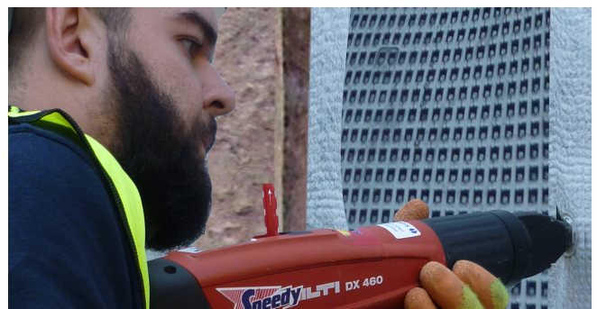
Fig. 6: Using a nail gun fix the Piledrain to each pile using stainless steel nails and plastic washers at 0.5m centres down each pile.
