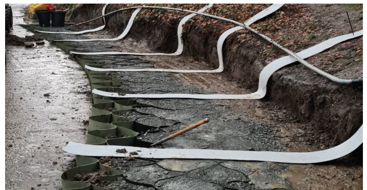
Fildrain drainage geocomposite strips positioned at 1m intervals from the back of the wall
