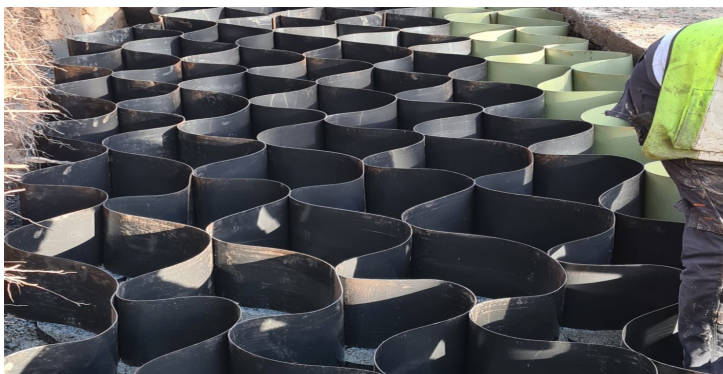
Type C Webwall panels expanded and pinned into position within the excavated footing
