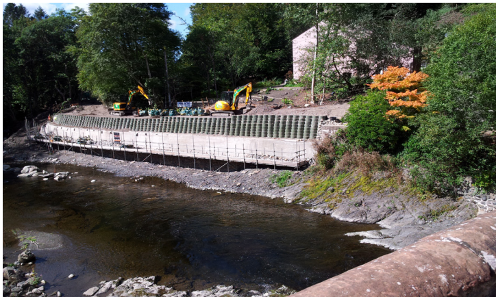
Designed to cope with flash flood levels
