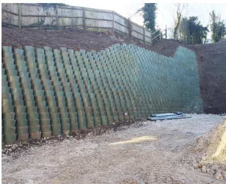
Webwall system reaching up to 8.25m tall at the far corner of the site
