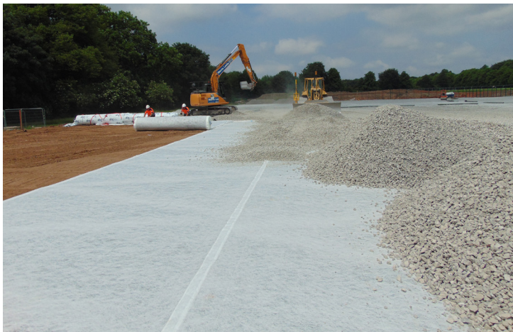
Rapidly installed large format rolls, simply rolled out across the formation and covered
