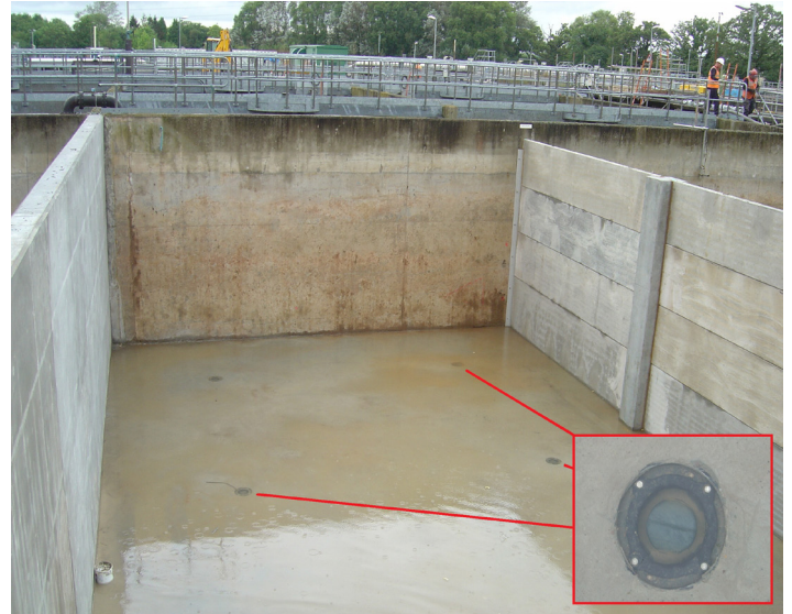
The finished floor slab with non-return valves for groundwater pressure relief when the tanks are empty
