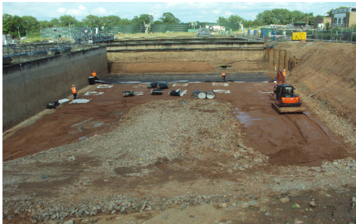
Placing Deckdrain with its geotextile facing down and the impermeable cuspatated face up ready to receive poured concrete
