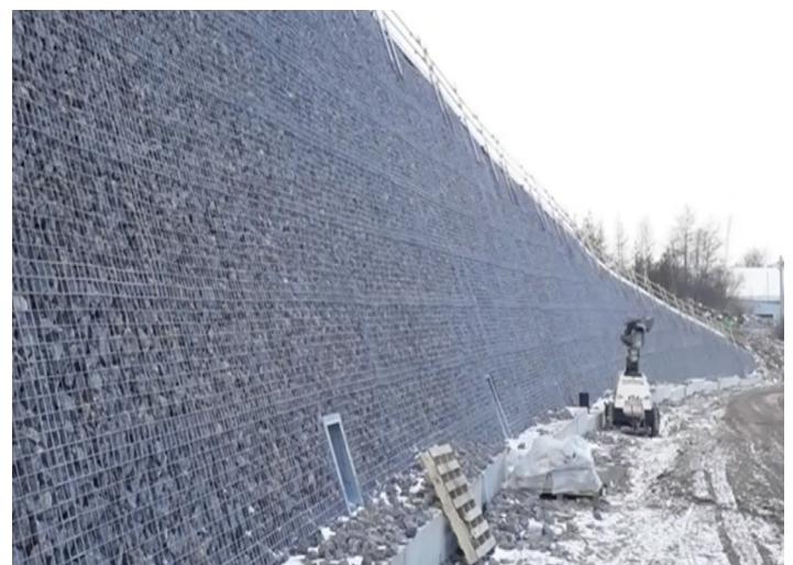
The finished SSTC rock/gabion style faced walls protected and drained with ABG Deckdrain.
