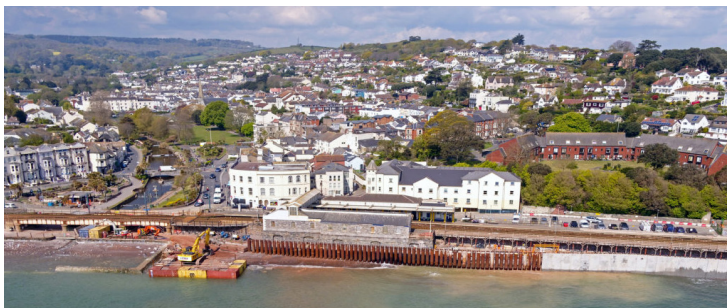
A section of the new, taller sea wall and promenade in front of Dawlish rail station
