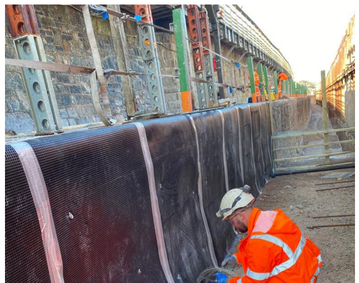
Deckdrain fixed to existing sea wall using Abfix pins & washers to maintain impermeability and jointing tape to prevent concrete ingress
