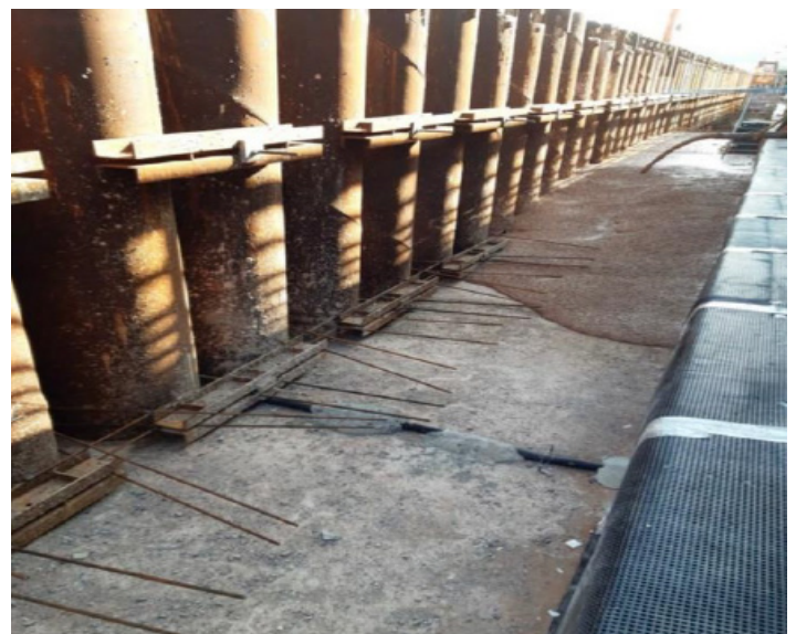
Concrete pour behind CHS pile wall. Deckdrain fixed to existing wall to channel surface & ground water from behind the new wall & promenade structure
