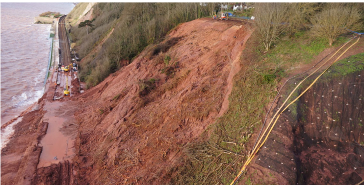
Land slide onto The South Devon Railway line following storms in February 2014
