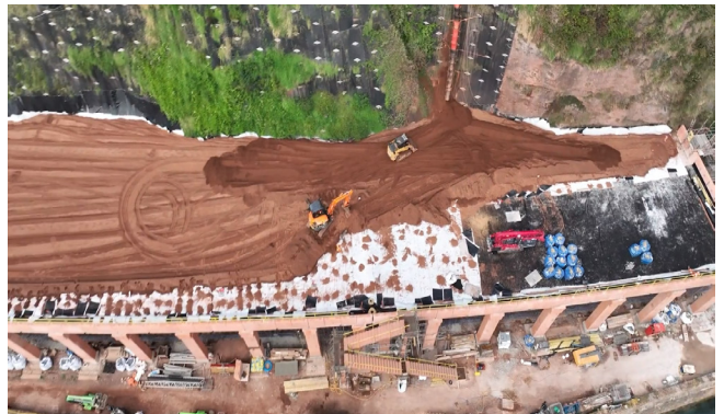
Deckdrain installed at the base of the cliff and onto the rockfall shelter roof and covered with red sand / soil mix
