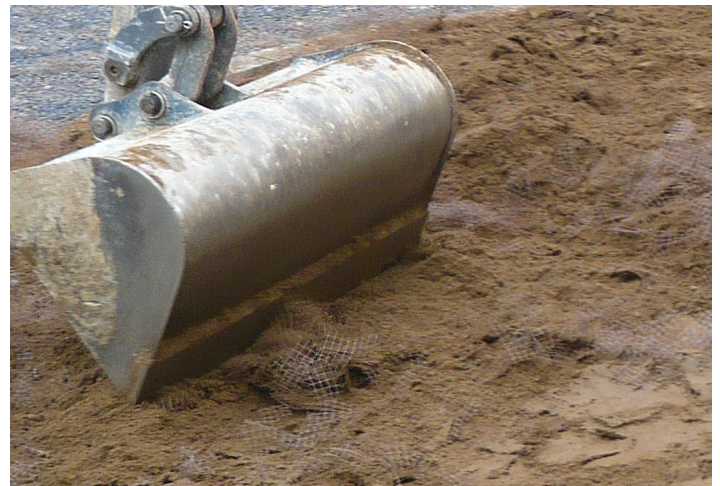
Advanced Turf System rootzone/mesh element blend (ATS400/B) being spread into access route areas
