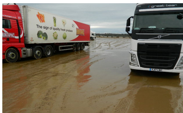
Poor condition of the truck stop HGV parking area prior to installation
