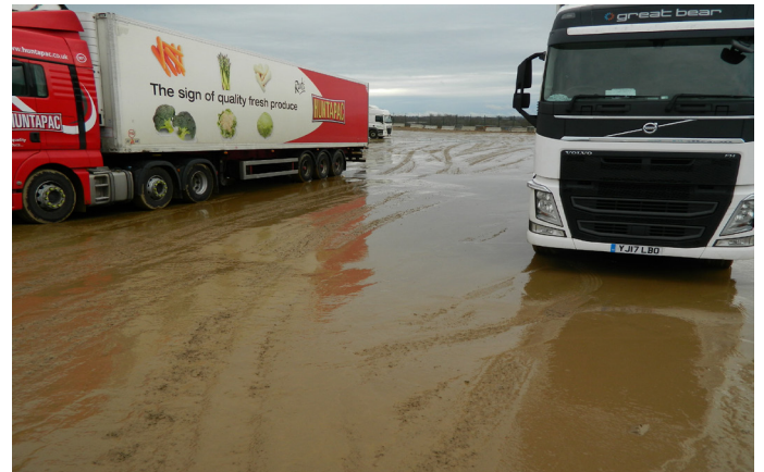
Poor condition of the truck stop HGV parking area prior to installation
