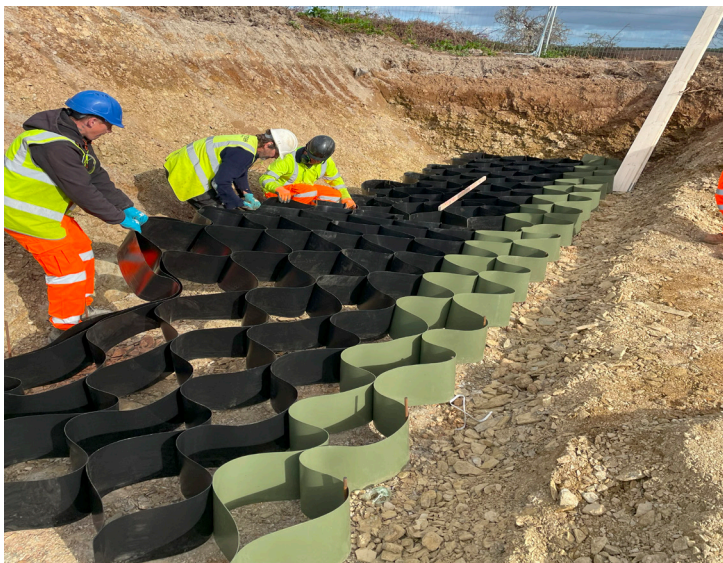
Setting out the first row of the Webwall by expanding the panel into position
