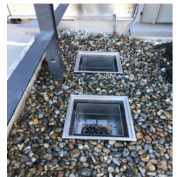
The bluerooF restrictor chambers
