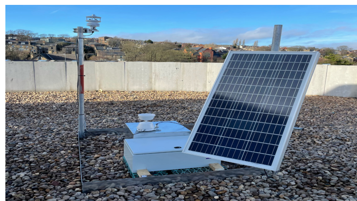
Rainfall monitoring station
