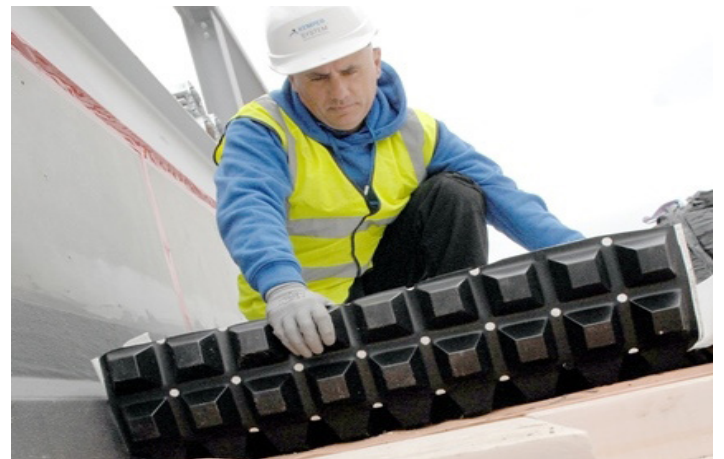
Placing the ABG green roof boards showing the overflow holes which then feed into the bluerooF attenuation system below
