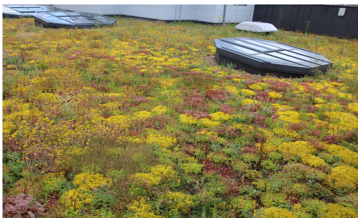
Mature sedum roof overlaying the ABG bluerooF attenuation system
