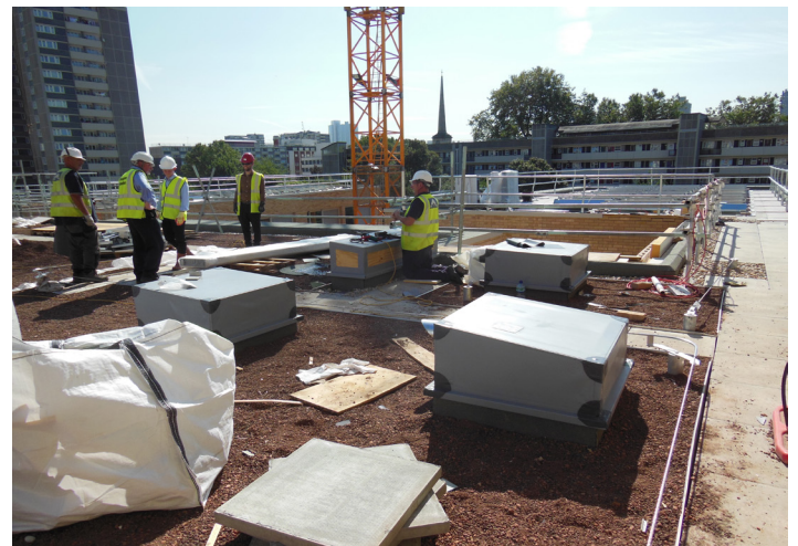
Biodiverse roof area during construction. Incorporated to enhance site ecology, contributing to the project achieving a BREEAM 'Excellent' Rating
