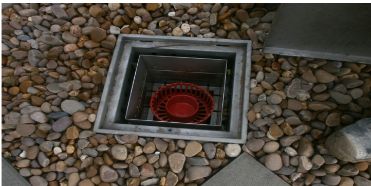
Stainless steel restrictor chamber over RWO
