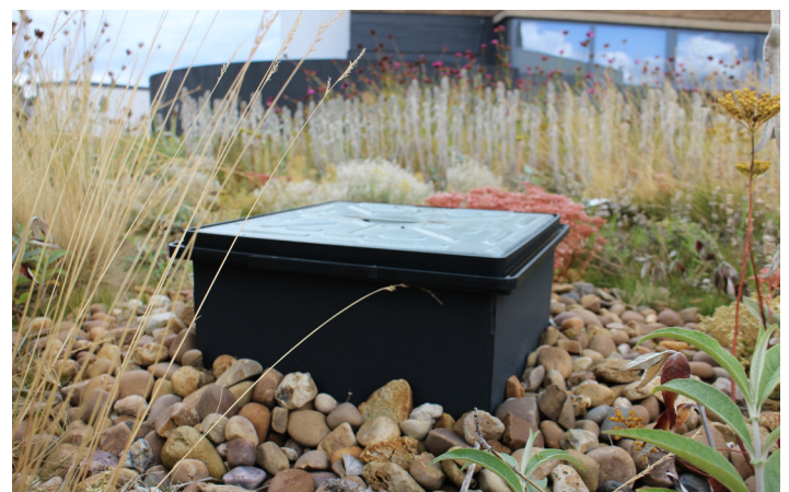
ABG bluroof restrictor chamber in biodiverse roof areas
