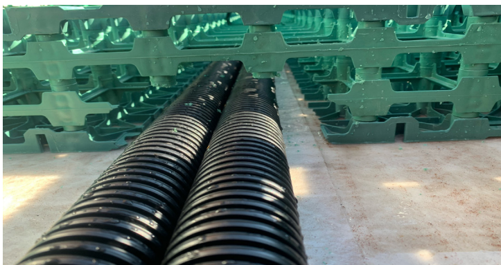
Cable ducting routed through the attenuation voids
