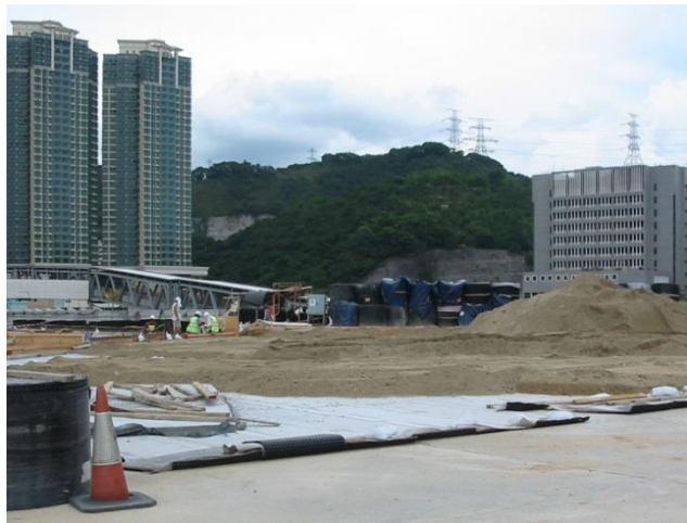
Deckdrain receiving cover layer up to 3m in depth prior to hard and soft landscaping, planting with trees and installation of innovative play areas
